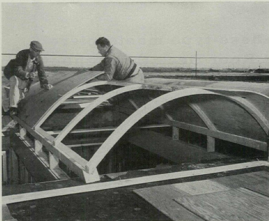
TOP SKIN is nailed to ribs. Note box beams under ends of the ribs.
