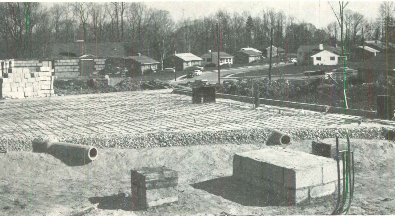
PHOTOGRAPH shows backfill around piers (foreground); warm-air ducts set in 6" washed gravel over fill; vapor barrier and mesh.
