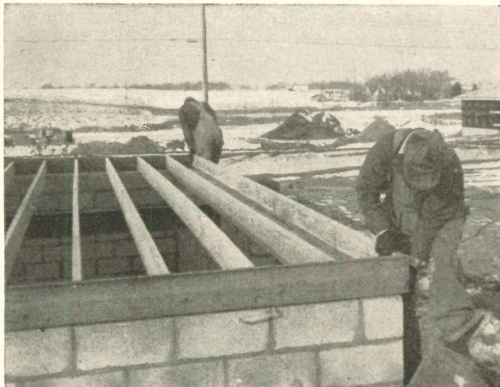
Crown in full-length joists draws down to beam when flooring and partitions are installed.
