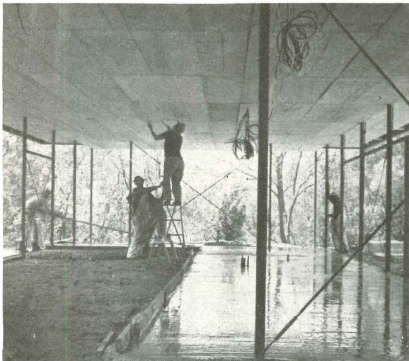
Construction was facilitated by 8' module. Plumbing, heating, under-slab wiring for floor plugs proceeded while framework was erected.
