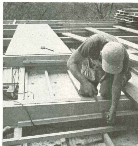
Ledger strips for roof panels took 1 1/2 man-days to nail. Steadier flow of prefab parts could have cut total on-site time to two weeks.
