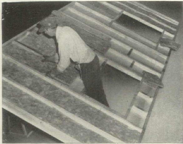
Fiberglas® Insulation being installed in wall panels at the National Homes plant in La Fayette, Indiana.
