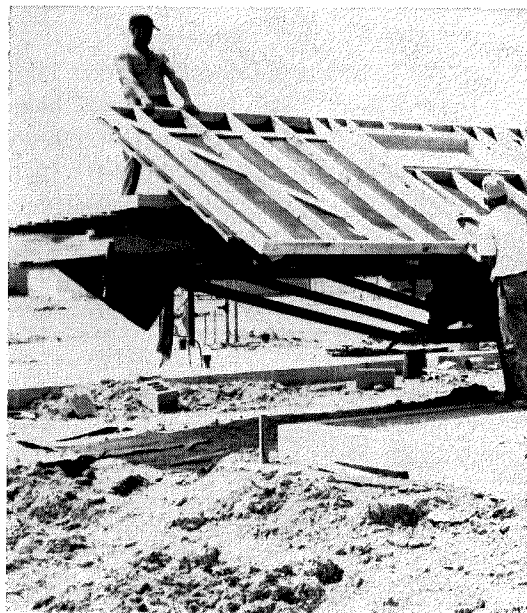
Exterior walls with one coat of paint applied are brought to job on special truck. Finished window frames are in place. Larger windows directly below top plate would have cost less.
