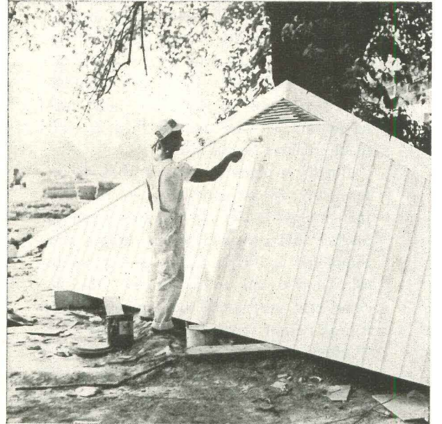
Point roller is used for both prime and finish coats. Here, gable end gets fast, efficient runover. Builders credit "controlled operation" allowing strict supervision of work and materials for the completion pace of two houses per day.
