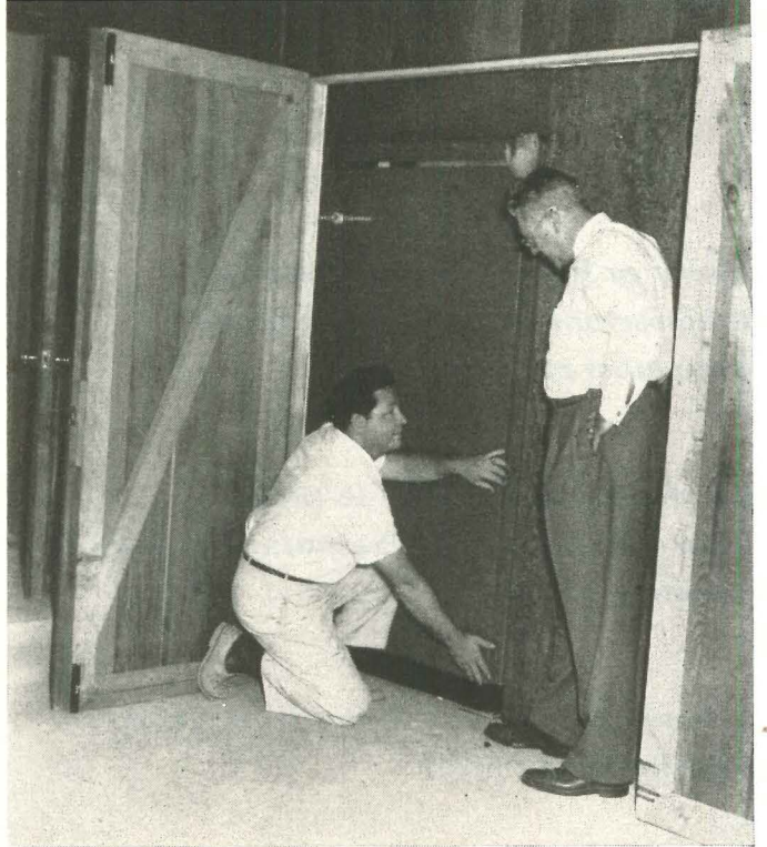
Valuable space inside house is conserved by putting heat pump outside. Thus ductwork for outside air circuit is eliminated; servicing is possible from three sides. Packaged 5 hp unit is 71" x 28½" x 37" high.
