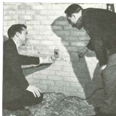
Weatherproof outlets are furnished at front and rear of house, eliminate makeshift arrangements for electric tools or outdoor Xmas lights.
