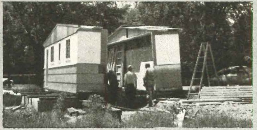
... Prefabricated panels and precut lumber stored in the units are used to complete the frame of the Knox-Bergstrom house when it arrives at site.
