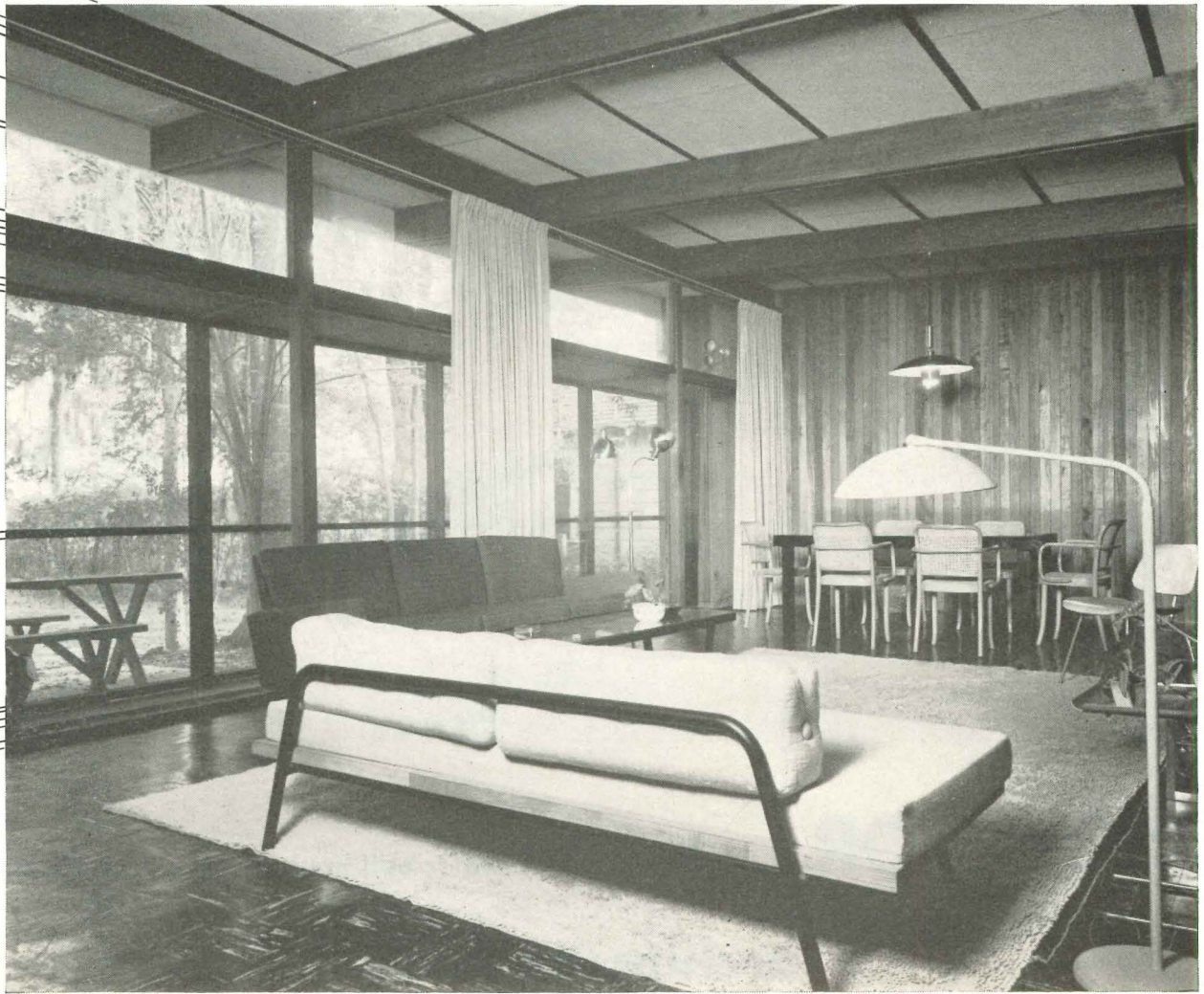
The roof structure is clearly visible in this picture: double redwood beams, steel purlins, cement and wood fiber board which also serves as the roof deck. Space between the screen cage and the sliding sash is part terrace, part plant bed.
