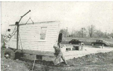
Builder who buys full-width panels with siding and windows may use mechanical cranes or large crews to install them.
