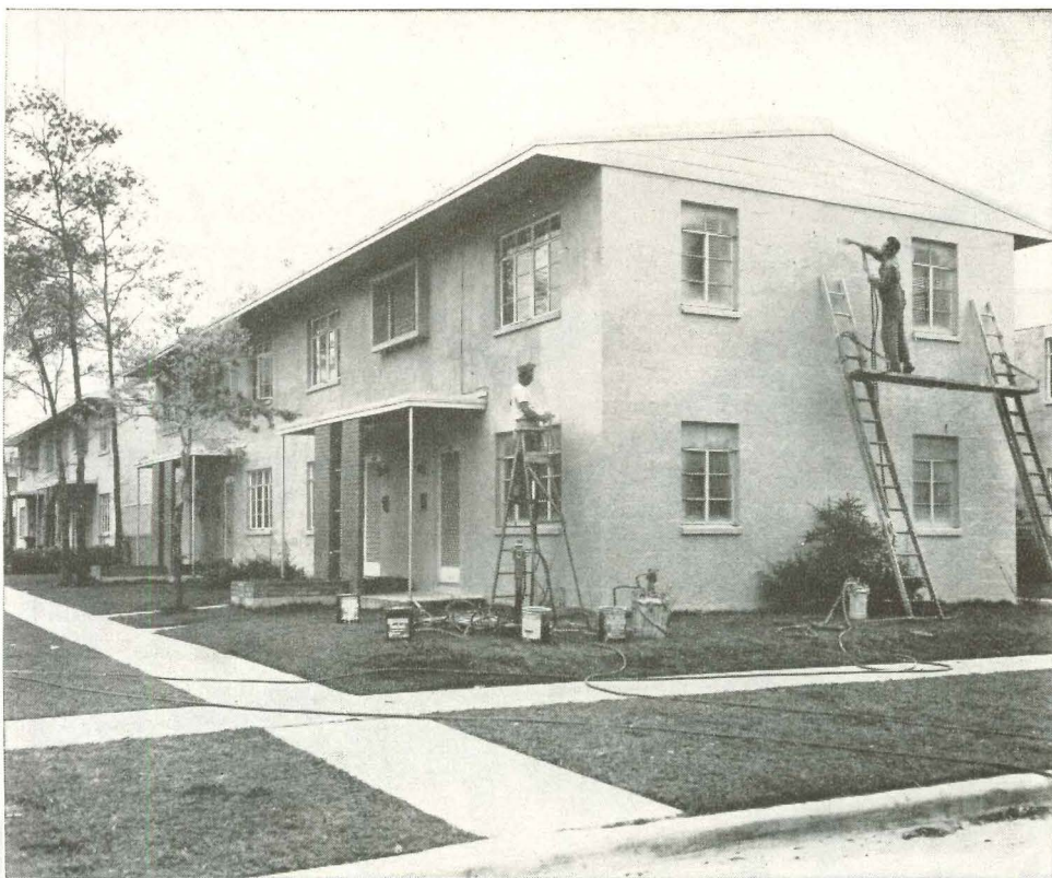
White vinyl plastic being sprayed over the cement block walls of apartment building.
