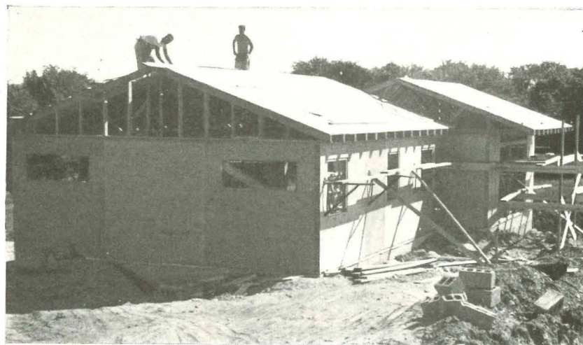
At the end of the day house is closed in by four workers. They put 1' x 8" sheathing on the roof. This operation speeded up with 1/2" plywood panels for sheathing. Trusses are on 2' centers local code forbids 1/2"
