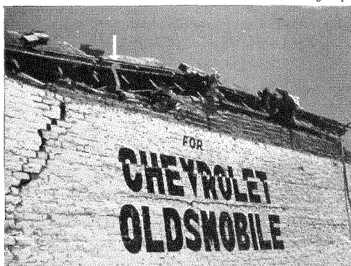
S-SHAPED FLANGES (arrow) one end of anchor bolts kept roof atop this quake-wracked brick wall, said building inspectors.
