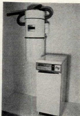
Receptacle for central vacuum system is mounted on wall in boots-and-parka closet, beside smokeless, odorless gas incinerator.
