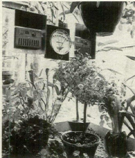
Dial of safety-alarm thermometer is flanked by heater and ventilator thermostats in metal hoods.
