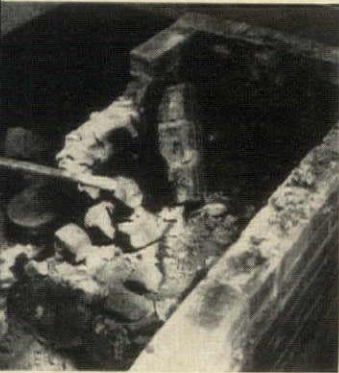
Old center bench was really a raised brick ground bed, had to be cleared by sledgehammer to make new floor space.
