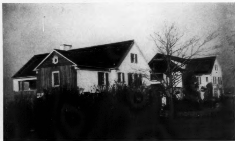
AFTER CUTTING THE OLD HOUSE APART, two separate houses were created. New end wall had to be added, two entrance drives laid out on the property. The north house had to have a new electric service cable and a sewer connection. But the interiors of both the houses were largely undisturbed. See pages 266, 285.
