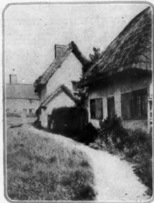
By its big projections at the eaves thatch roofing is able to protect the walls from the weather. The material on these cottages at Rye, England, is straw
