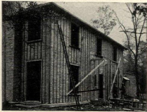
House near Chicago, showing its "underclothing" of Cabot's Quilt with furring strips over Quilt, on which outside finish is laid. Roof also insulated. Russell S. Walcott, Architect, Chicago, Ill.
