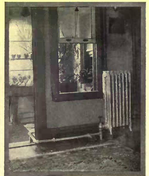
By elevating the radiator, a water pocket was avoided and the proper drainage assured
