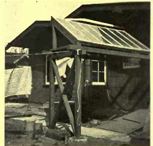
A solar water-heater mounted on the roof and supplying water at a temperature of 100 deg. F.
