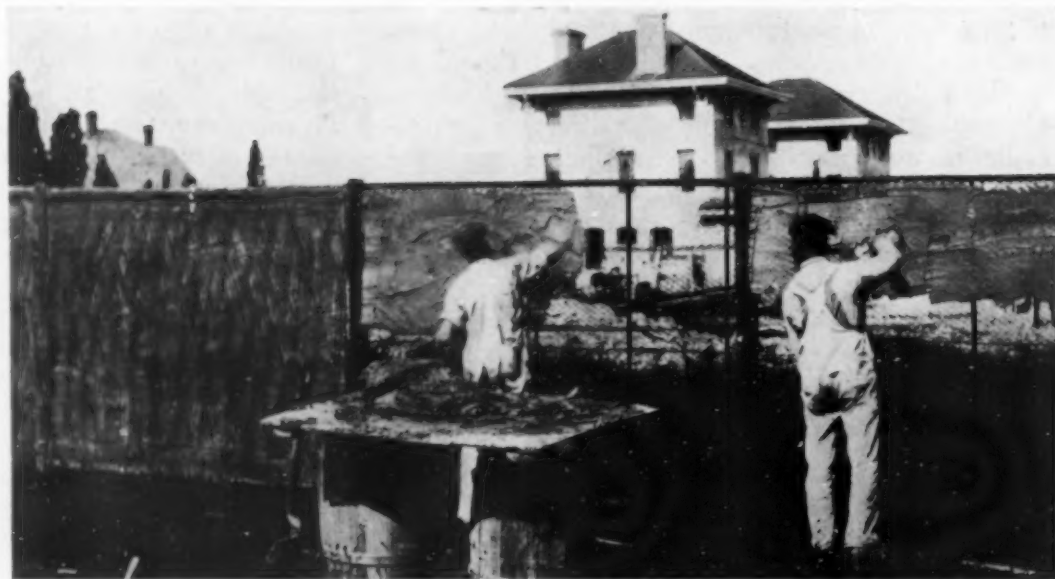
Fig. 7. Making a cement fence with expanded metal. The latter is plastered with cement mortar, making a cheap but desirable fence
