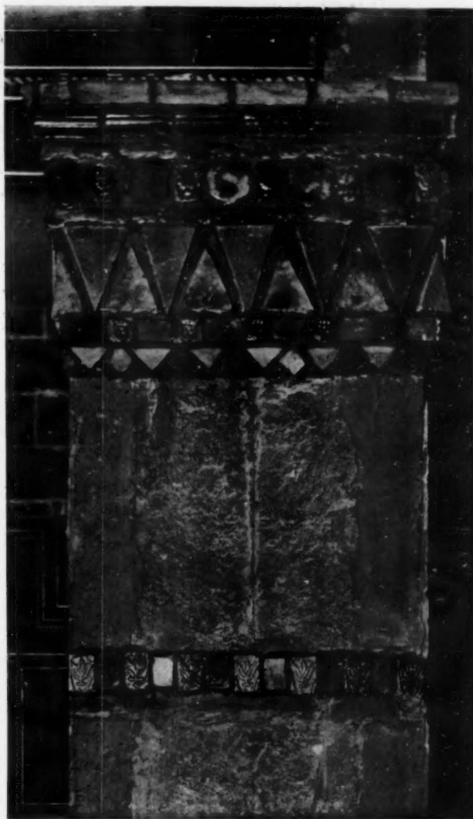
Fig. 3. Concrete column in original rough state, decorated with a capital set in the concrete consisting of flat tiles, glazed and unglazed. Colors: green, red, brown, yellow, blue and buff. The lower band of tiles has been inserted in a groove chiseled in the finished column
