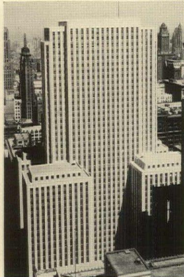
Aluminum spandrels and windows are installed in the Field Building, Chicago. Architects were Graham, Anderson, Probst & White of Chicago.
