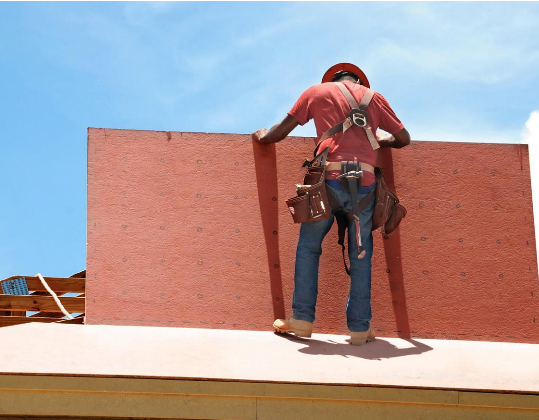
Providing an air barrier as part of the roofing sheathing is one way to assure continuity and effective performance of the roof.
