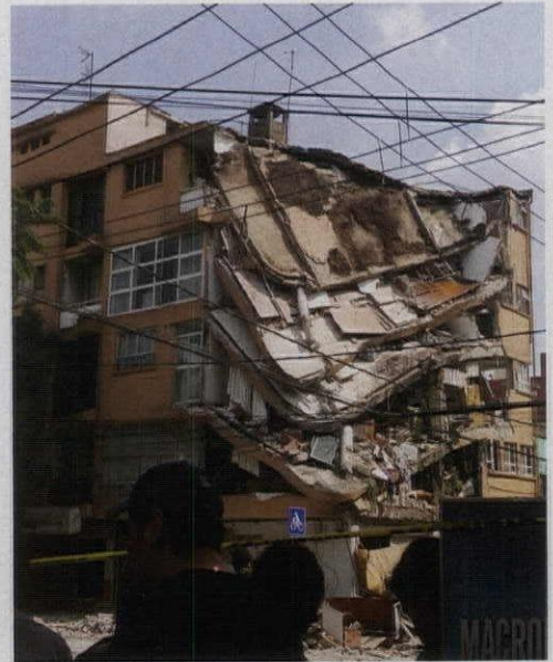
The September 19 earthquake also wreaked havoc on many neighborhoods of Mexico City, including Colonia Narvarte, pictured here.
