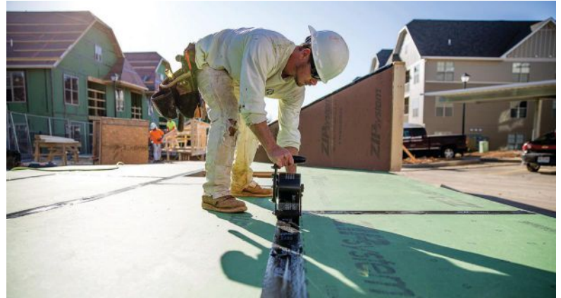
Installers pre-assembled ZIP System® sheathing panels and tape before installing on exterior walls and roofs.
