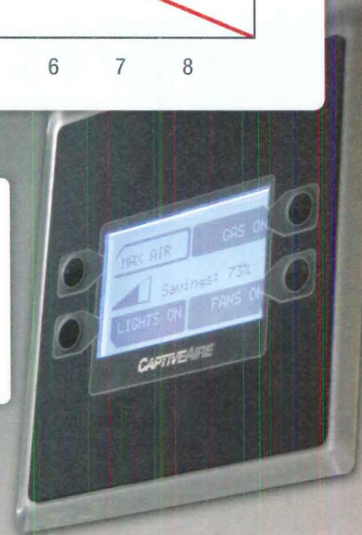
Electrical Controls with LCD Screen
