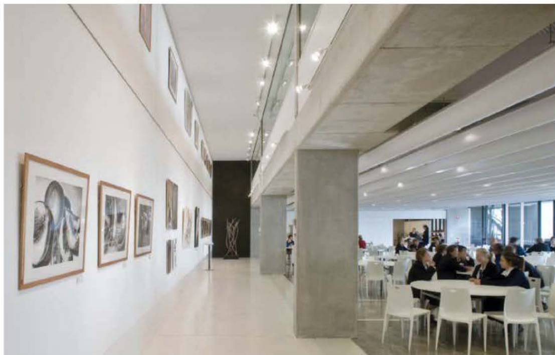
Billowy fabric ducts on the ceiling of the cafeteria at the Brisbane Girls Grammar School help mitigate the acoustically undesirable characteristics of the mostly exposed concrete structure.
