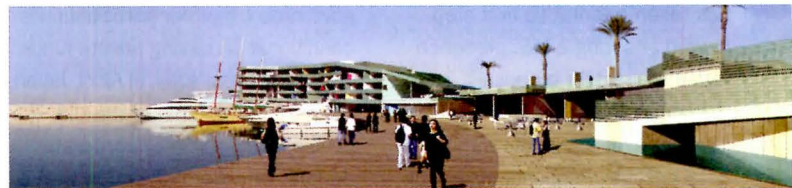
Excavation has just begun on Beirut's new marina, by Steven Holl and L.E.F.T.
