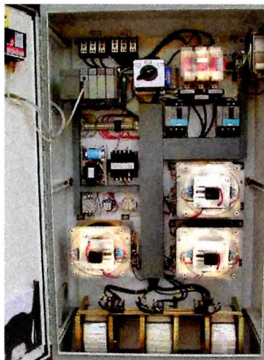
Inside a PowerTec dimming system.
