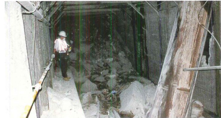
The 1/9 (top two) and N/R (above) subway tunnels incurred significant damage on September 11. Cost estimates to rebuild have not been announced.
