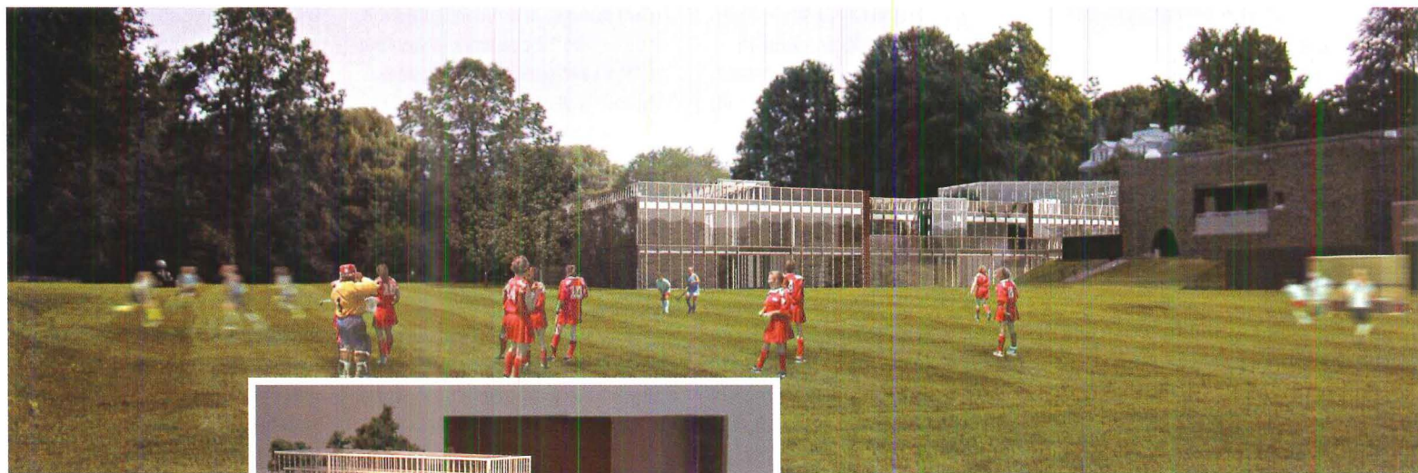
Now under construction, SOM's new upper school for Greenwich Academy in Connecticut has five disciplinary clusters set between a lake and green fields.
