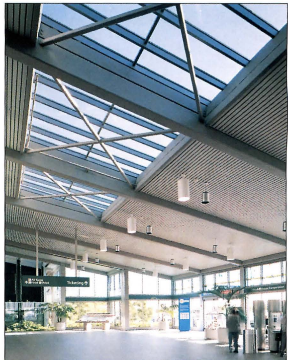
Photo: Sacramento International Airport, Terminal A Architect: Dreyfuss & Blackford Architects Photo: Cathy Kelly Architectural Photography A/D FIREFILM® II on structural steel.
