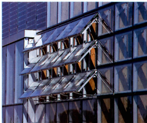
Building openings (left) are controlled by a computer system that monitors indoor and outdoor temperatures. There is no air conditioning. PV panels, clustered in varying densities on the roof (right), create cloudlike patterns below. There are no panels over the center atrium.
