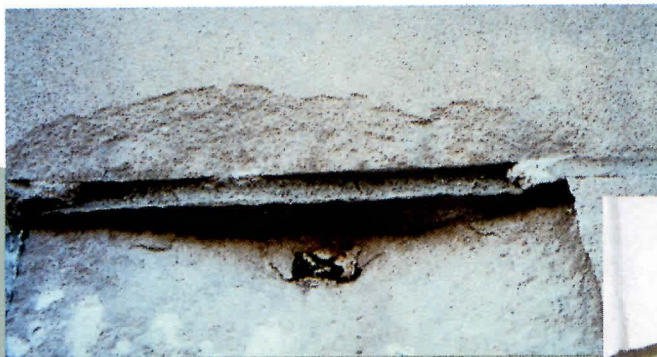
THE STONE IS SPALLED AT SOME JOINTS where ties bind the expanding masonry to the shrinking steel frame (above). Test panels were cleaned using nondestructive methods (right).
