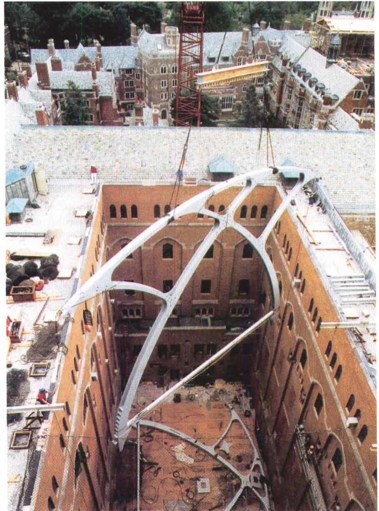
Shepley Bulfinch Richardson and Abbott designed a neo-Gothic truss for a Yale library with an eye to installation logistics.
