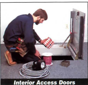
Interior Access Doors
