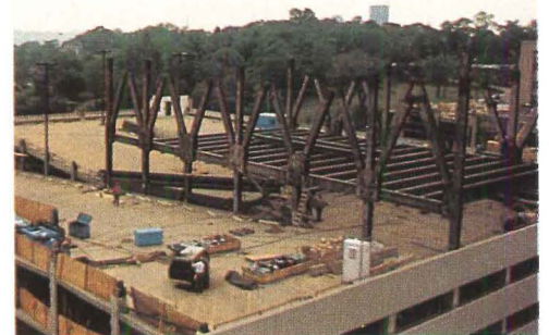
The Presbyterian-University Hospital Tower (middle) rises 21 stories. Installation of transfer trusses at the Biomedical Sciences Tower (above).
