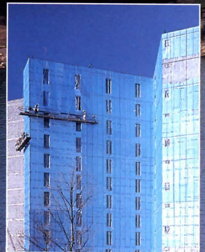
FULTON COUNTY JAIL, Fulton County, Georgia Now under construction Ova, Daniels, Busby — Architects
