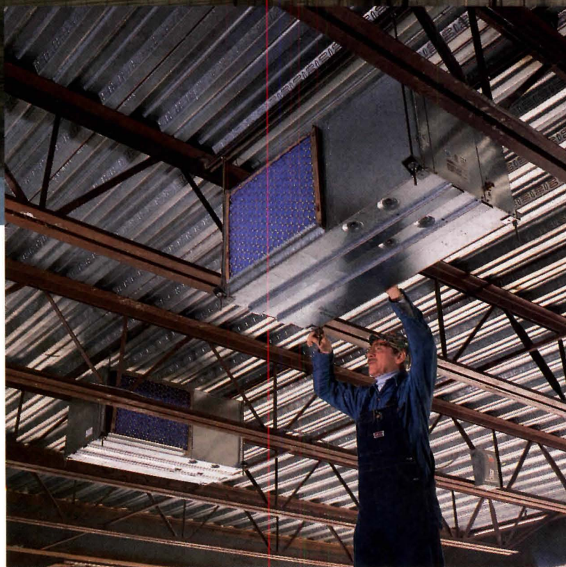
5-foot spacing between Vulcraft joists permits easy installation and maintenance of heat pump units.
