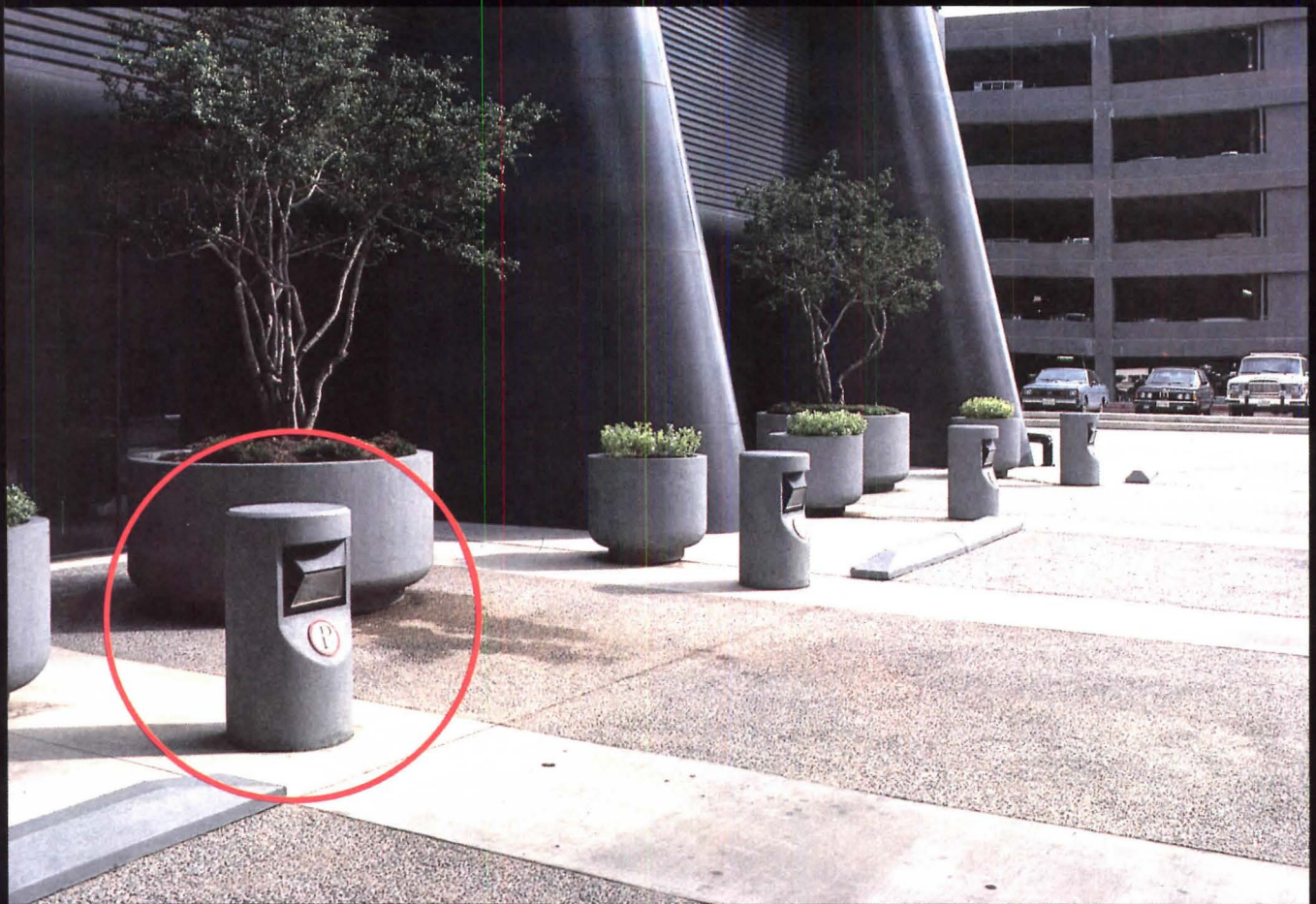
Kim Low Level Floodlights in precast concrete pedestals.
