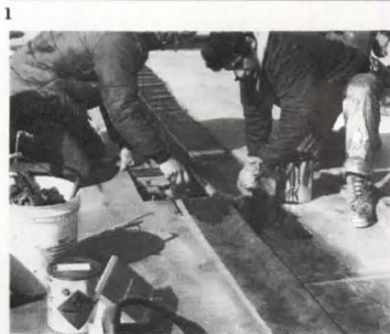
2 Stress forces, as shown in the drawing above, challenge roofers to make their field seams with care. Shear stresses, caused by expansion or contraction of a building or the movement of insulation materials or other substrates such as decks, can deform seams, subjecting them to peel forces as well—to which they have less resistance. The
