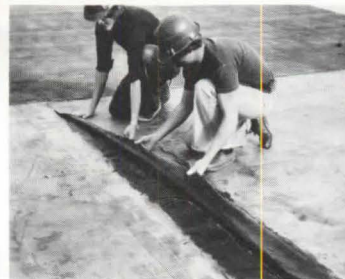
3 photo 2 at left. But before this step, the roofers first treated the EPDM membrane with the adhesive-promoting primer mentioned earlier. In a conventional seaming operation (photo 3) roofers join the laps after the solvent in the contact adhesive has “flashed off” and the adhesive has dried. The laps of a specially processed talcless EPDM
