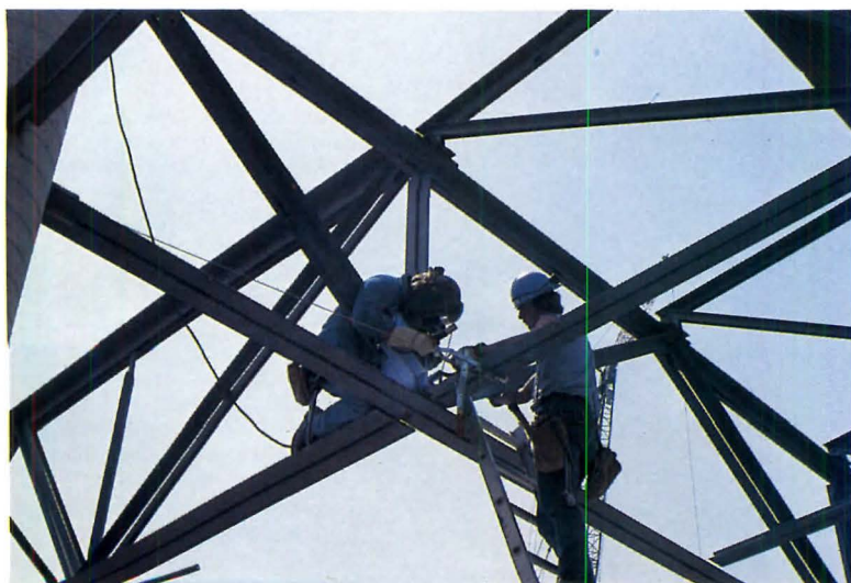
The uniform depth of the steel joists and joist girders added important aesthetic qualities to the arena.
