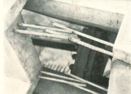
Galvanized steel rebars near surface of seat-base units.
