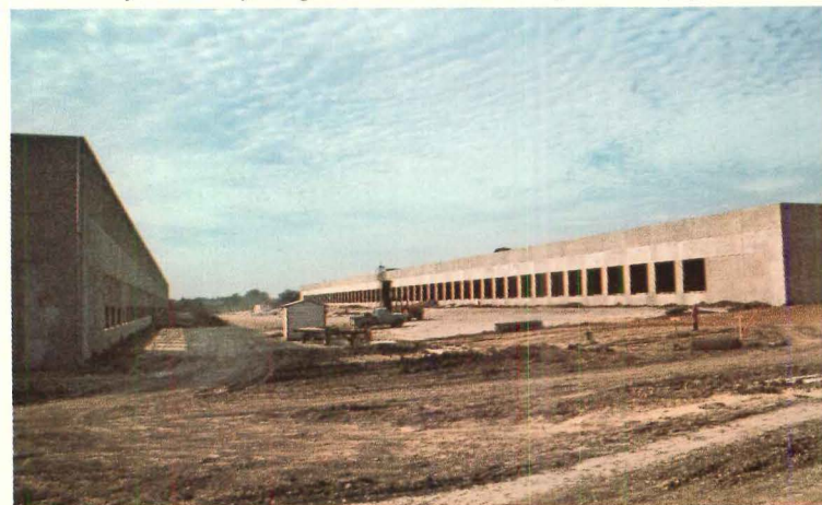
Ease and speed of erection with Vulcraft products enabled the first building to be under roof in 19 days.
