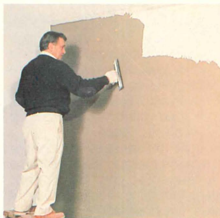
with its factory laminated fiberglass mesh, is applied to the gypsum board. In the second photo, the strong, cementitious prime coat is troweled over the insulation. And in the third photo, the
