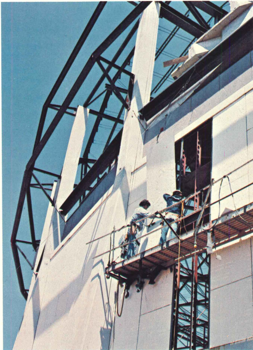
Exterior walls of the new Huntsville, Alabama, Civic Center are J-M Stonehenge® architectural panels secured directly to the steel studs. Here insulation is sprayed on the back of the panels. A combination of hidden and reveal joints was chosen by the architect.
