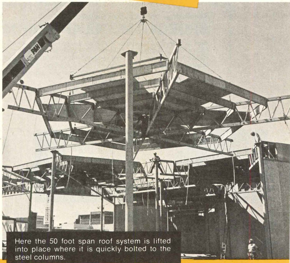
The TJ space frame (modular hexagon pods) is constructed on the ground where it goes together quickly and easily for big labor savings.
