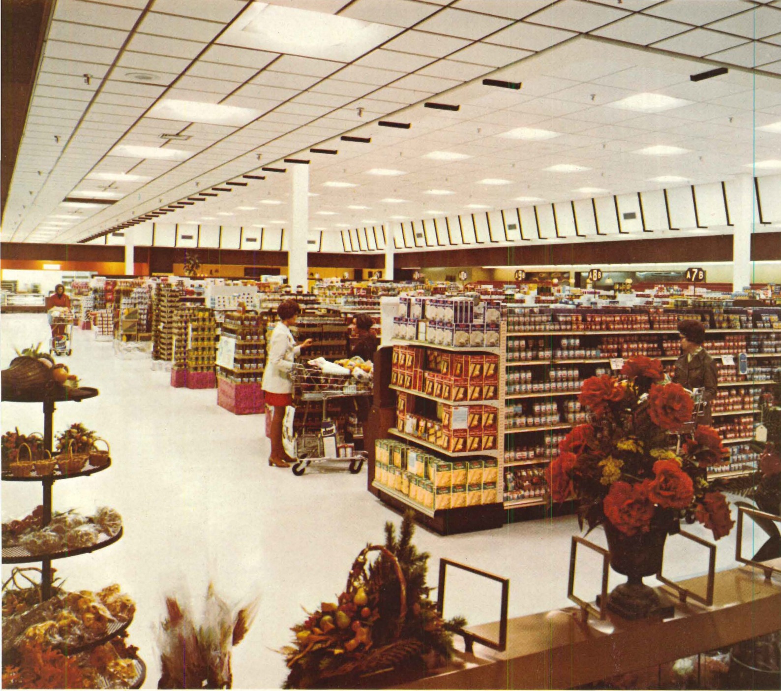
GE Lowmount Regressed enclosed luminaires provide ideal supermarket illumination.
