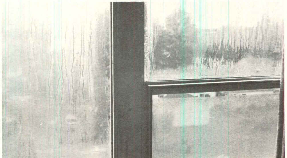
Condensed moisture within the air space—a sure sign that the insulating glass seals have failed.
