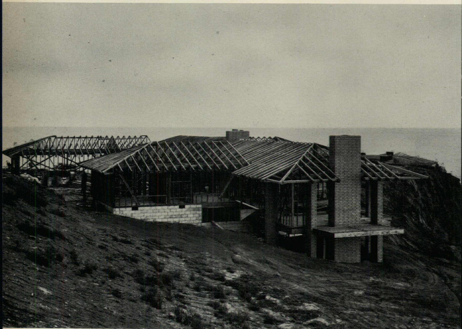
Kermit Dorius, A.I.A., 5000 sq. ft. residence for W. T. White III, Laguna Beach, Calif. 19 special trusses designed plus trussed floor systems.
