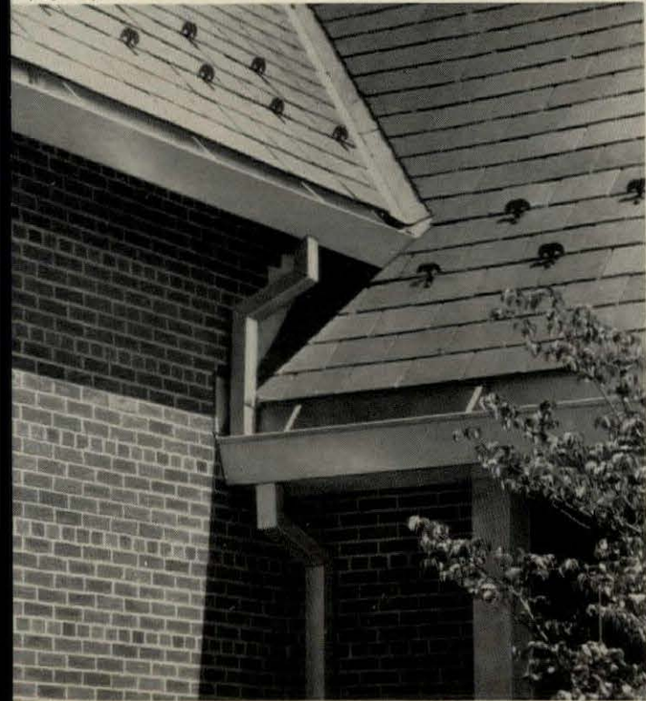
STAINLESS STEEL VALLEY FLASHING, valley flashing, gutters, downspouts, roof flashing and chimney flashing. Trinity Episcopal Lutheran Church, Latrobe, Pa. Architect: Mansell-McGettigan Co. General Contractor: Pevarnik Brothers. Roofing Contractor: Miller, Gas, Gyekis, Inc.
