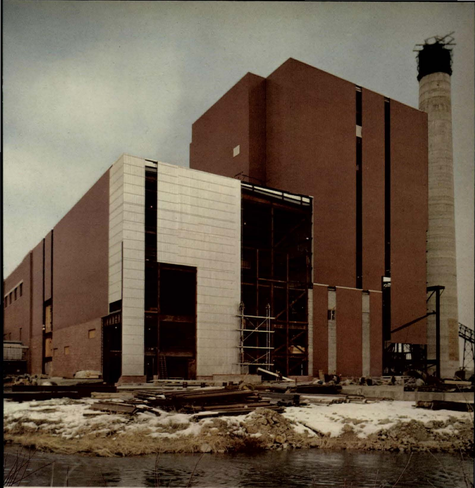
Trenton Channel Power Plant, The Detroit Edison Company, Detroit, Michigan
