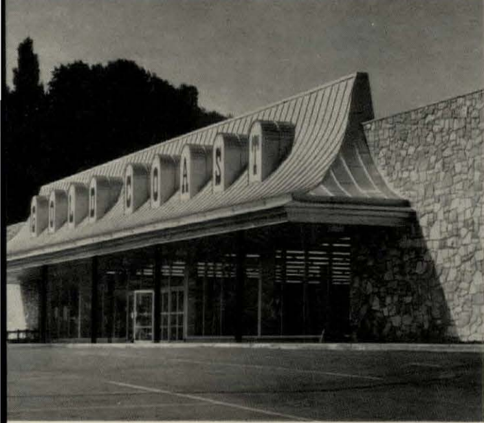
STAINLESS STEEL standing seam roof, valley flashing, fascia, gutters and downspouts. The Gold Coast, Maitland, Pa. Architect: Lucian Caste. General Contractor: Caste Development Co. Roofing Contractor: General Roofing Co.
