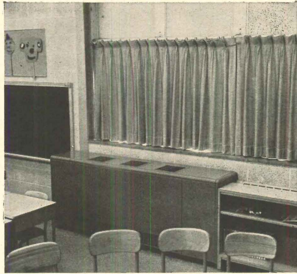
Typical gas heating unit.
