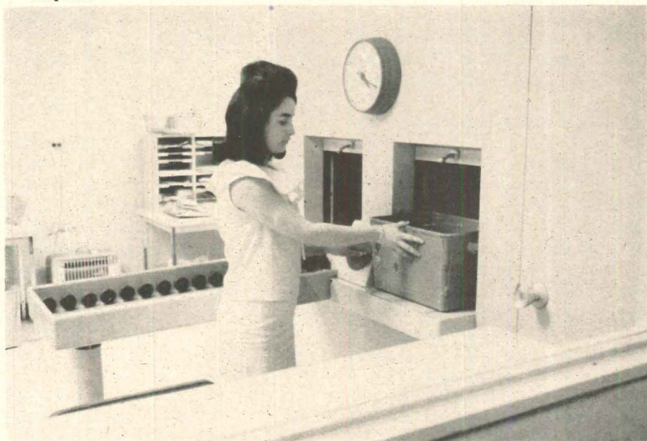
A service mail room on the 15th floor of the Penney building. Trays are dispatched on the right and delivered on the left; the floor selector is between the hatches.
