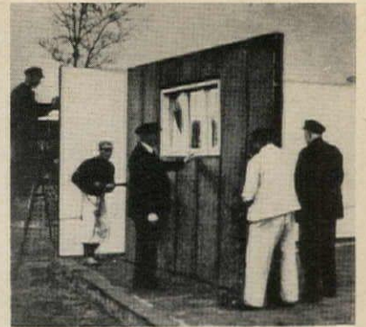
Erecting a prefabricated house designed by Walter Gropius in the Bauhaus years
