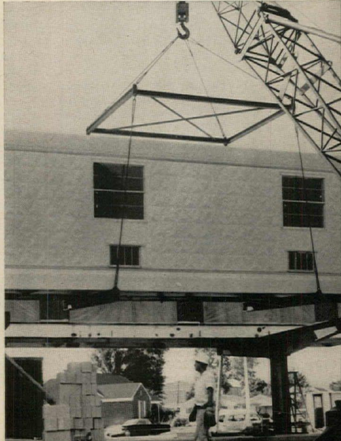
A four bedroom section being swung into position by crane. Two duplicate sections, facing a corridor, provide a total of sixteen rooms.
