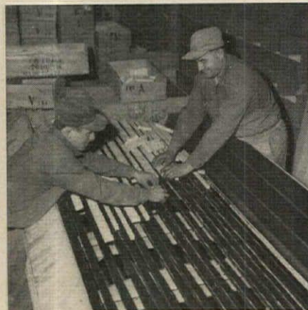
Marble pieces are fitted into the rubber extrusion form by hand. Concrete will then be poured into the form and vibrated to insure a close lock with the grooved marble strips
