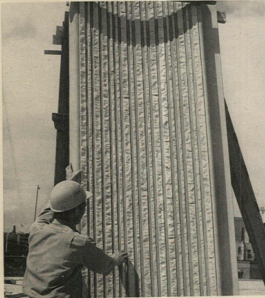
Each precast concrete panel for the Toronto City Hall (scheduled for completion in 1965) has strips of split-faced marble set into it. Special techniques were developed for molding the marble strips into the panels. The building was designed by Viljo Revell, of John B. Parkinson Associates, Architects & Engineers, Toronto, Canada
