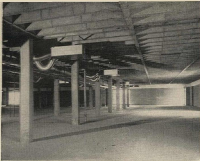
Dual-duct air system on unfinished floor of the academic wing
