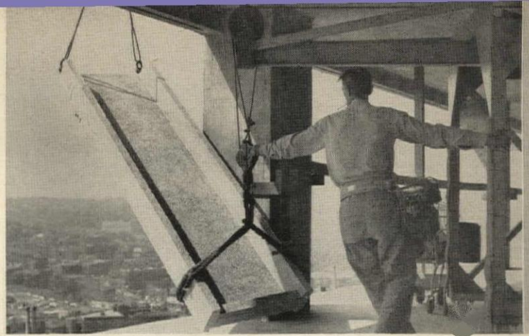
1 A Mo-Sai curtain wall panel being hoisted into position ready for anchorage.
