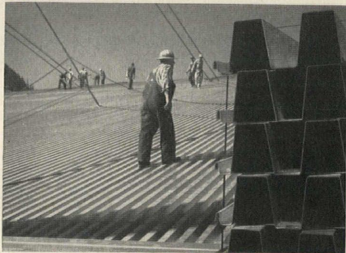
Deep-formed Bethcon sheets were welded to flat sheets to form unique cellular units designed to carry warm air for heating and snow removal.
