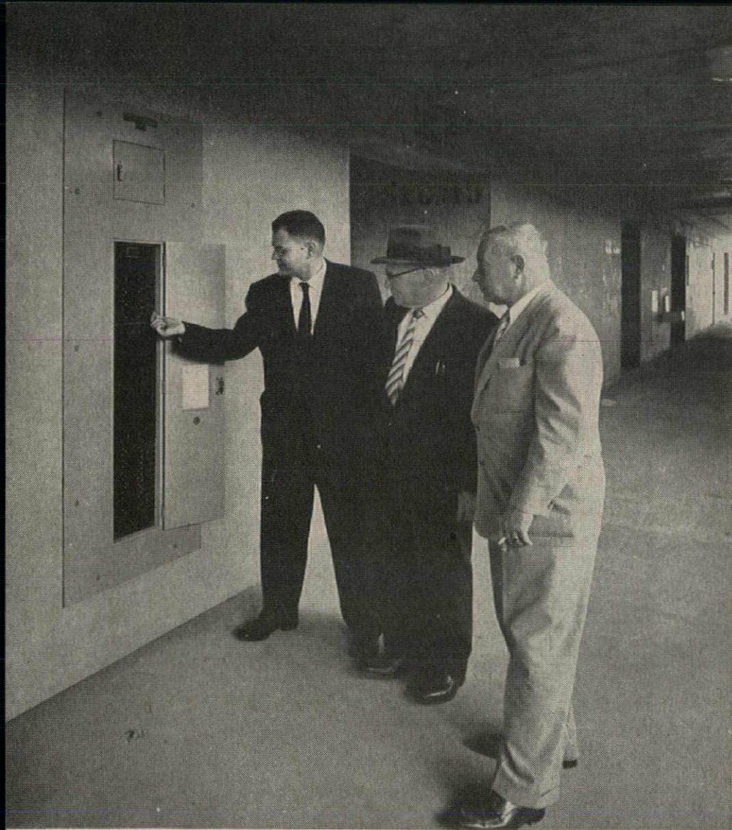
Lighting for concourse and corridors is controlled and protected by Type NLAB panelboards located around stadium. Relays and control switches installed in this panel allow remote operation from centralized point. Seen examining this attractive flush mounted panelboard in stadium concourse are H. G. Dechene and G. R. Brayer of Brayer Electric Co.; and Spence Pors, Westinghouse Distributor Salesman.
