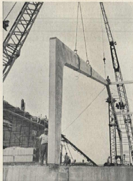
As one crane raised and held the 18-ton arch half, another (on the right) guided it into position. The two halves were then welded together to form complete arch.
