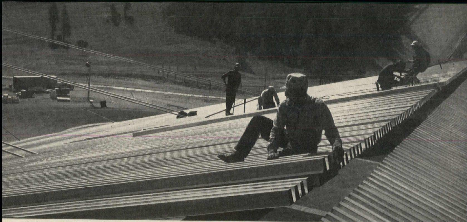
Roof under construction at Squaw Valley Winter Olympic Ice Arena. Associated Architects: Corlett and Spackman, A.I.A., and Kitchen and Hunt, A.I.A.; Structural Engineers: H. J. Brunner, San Francisco, and John Sardis, San Francisco. General Contractor: Diversified Builders, Inc., Paramount, California.
