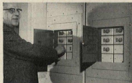
G-E master selector switches at ends and center of each floor control lighting separately for each 1/2 floor. Building contains 2000 fluorescent lamps.
