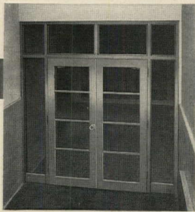
Overly U/L Labeled Fire Barriers
