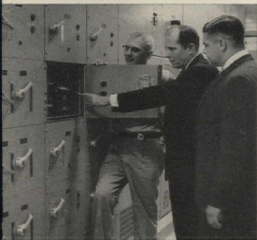
Jacob Dietrich, Building Engineer, Bankers Life of Nebraska; A. J. Whitmer, President, ABC Electric Company, Electrical Contractors; and W. F. Sterbens operate pushbutton of one of the combination Life-Line® starters in the motor control center portion of the 1500-kva power center. This control center feeds, protects and controls all motors and feeder circuits in mechanical equipment room.
