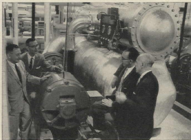
One of two Westinghouse 200-hp Life-Line motors which drive compressors in air conditioning system. Westinghouse motors from 1 to 200 hp were specified for all auxiliary equipment drives. Having a single source of supply simplifies maintenance and spare parts problems for operating equipment. Discussing the installation are J. P. Anderson; C. E. Pickering; J. O. Unthank; and Harold Stebbins, Vice President, Bankers Life of Nebraska.
