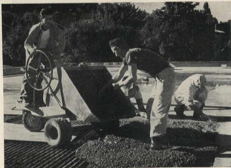
Pouring is no problem with Fab-Form. Here a buggy has rolled over Fab-Form without damaging the material. Six-inch square mesh made of No. 6 gage wire is from Pittsburgh Steel, too.
