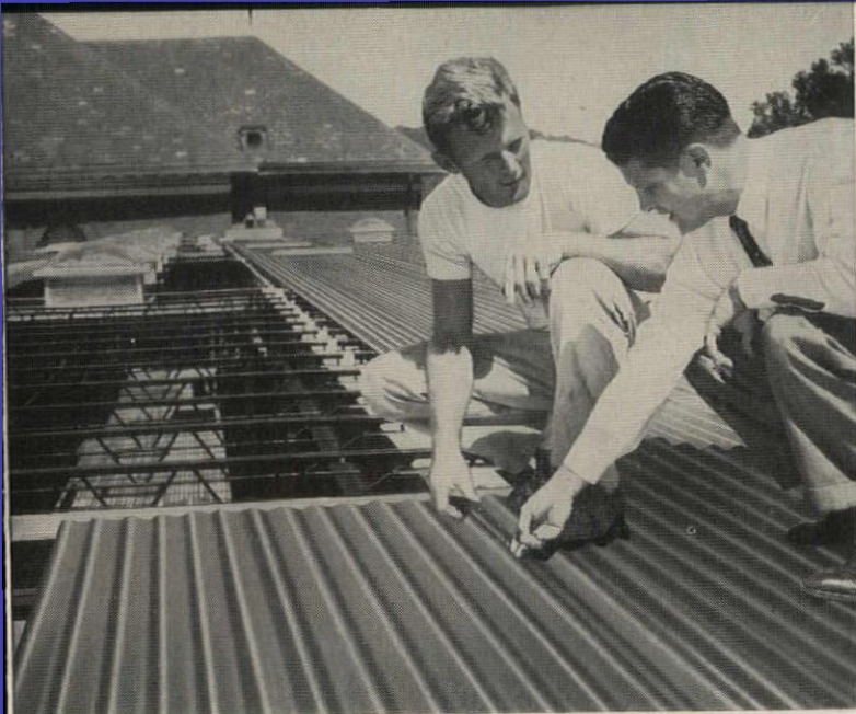
Deepest corrugation , \frac{5}{8} -inch, of all standard steel centering is available with Fab-Form. Job Superintendent Thomas A. Laboon, left, shown with Pittsburgh Steel Products Salesman C. W. Bainbridge Jr., said deep corrugation helped make a stronger slab.
